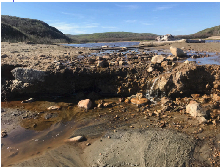
Exposed abandoned sewer line February 11th
